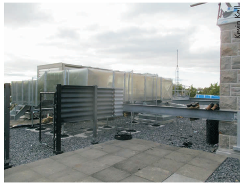
The AC area adjacent of the rooftop observing deck.
