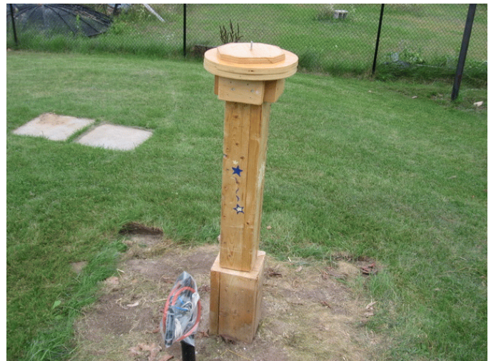
The 2"x4" pier is inserted into another 2"x6" pier that was already in the ground and cut short.
