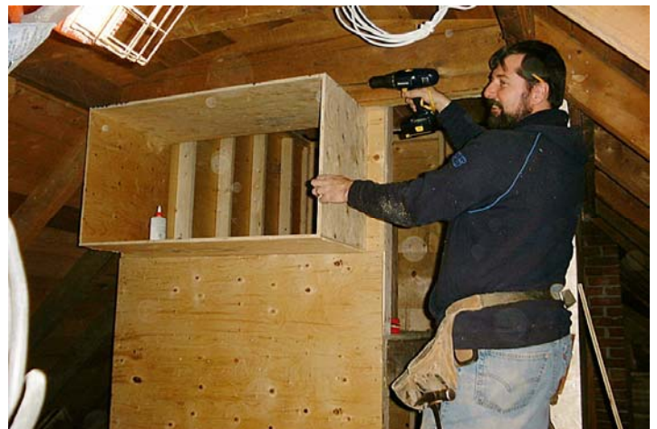
A storage cubby was built into the north wall of the observatory. Since the observatory interior is only 6'x6', the storage space is quite handy!
