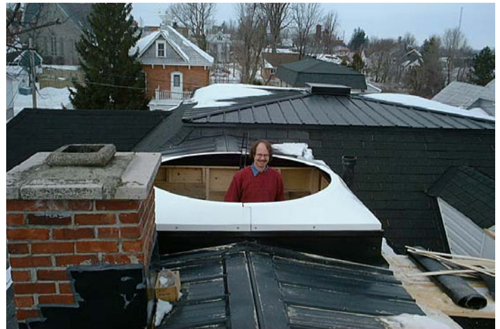
On top at last! Standing on the observatory floor and looking around the opening in the roof for the first time was the highlight of the construction phase for me!
