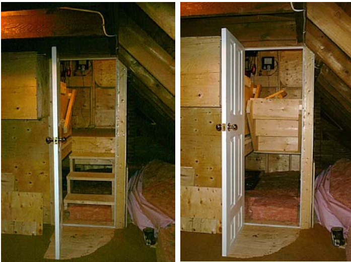
The stairs are hinged to allow flipping them up out of the way to give access to the volume underneath the raised floor. This is handy when running new wires out to the dome!
