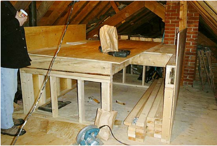
The raised floor of the observatory, including the cutout (at right) for the stairs.
