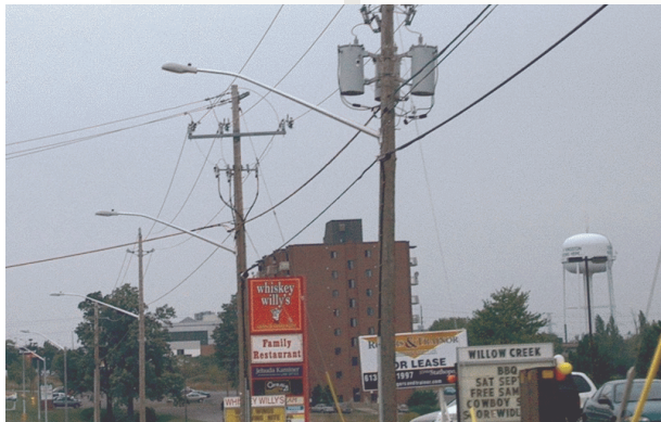
New street lighting along Gardiners Road in Kingston... with Full Cutoff Fixtures! Yay!
